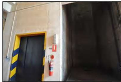
Figure 48. View of the crane well centralised between two service lifts. Only one lift is in view. (Source: Heritage 21, 09.03.16)
