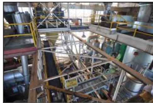
Figure 44. View looking down of the roasting hall from fifth floor platform. (Source: Heritage 21, 09.03.16)
