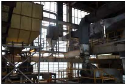
Figure 45. View looking up of the roasting hall from fifth floor platform. (Source: Heritage 21, 09.03.16)
