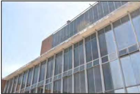
Figure 49. View of clerestory aluminium framed glazing as viewed from the second-floor roof space.
