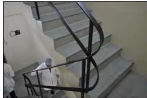
Figure 50. Curved steel handrails located in stairwell located between floor five and floor three. (Source: Heritage 21, 09.03.16)
