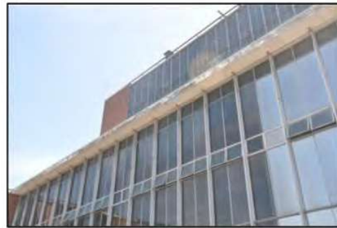
Figure 46. View of clerestory aluminium framed glazing as viewed from the second floor roof space. (Source: Heritage 21, 09.03.16)
