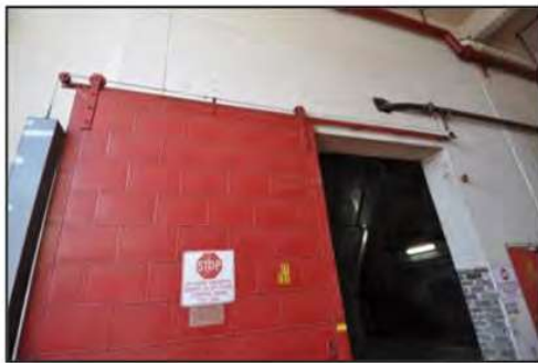
Figure 47. View of sliding steel fire escape door located on the second floor. (Source: Heritage 21, 09.03.16)
