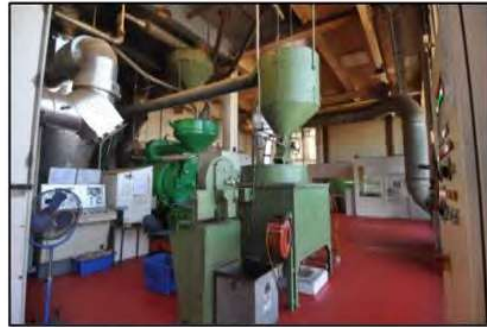
Figure 44. Detail of space and equipment located on second floor.
