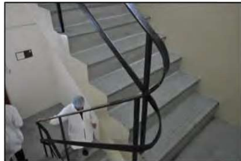
Figure 42. Curved steel handrails located in stairwell located between floor five and floor three.
