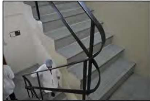
Figure 50. Curved steel handrails located in stairwell located between floor five and floor three. Despite not achieving BCA Compliance, the existing handrails should be retained and reused on site.
