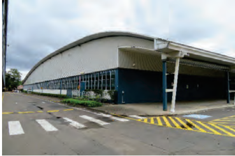
Figure 2.5 View of the west elevation and rear corner of the building, showing the arched roof and one of the covered loading bays.
