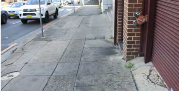
The existing condition of the footpath along Victoria Road is in need of replacement
