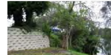
Embankment infested with weeds and dead or dying trees (8)
